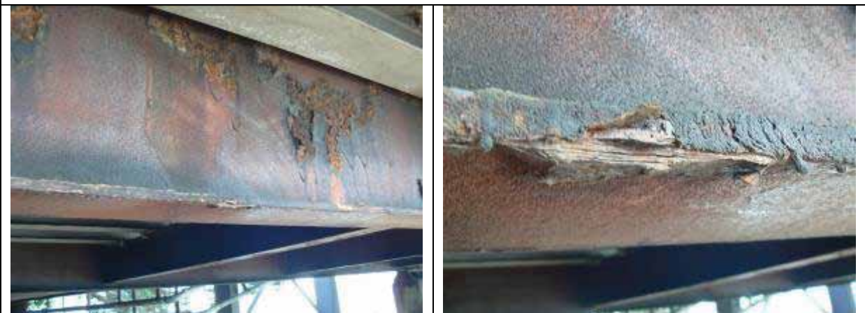
Chelsea Wharf – coating under Gold Seal exhibiting cracking and flaking on I-beams.
