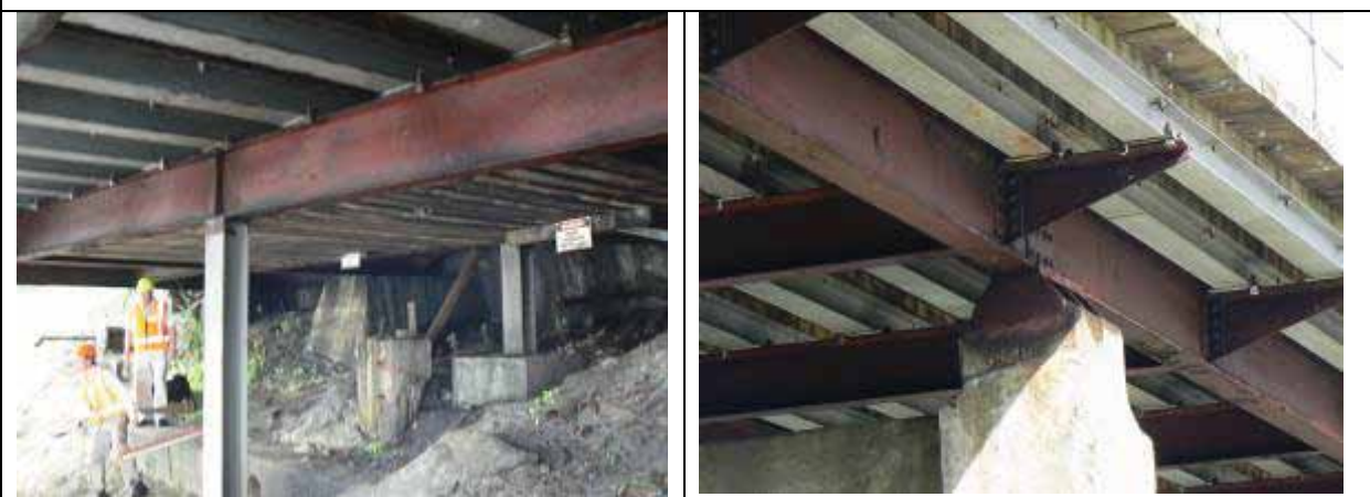
Chelsea Wharf – I-beam construction, Gold Seal coating not reinstated After 2006 modifications.
