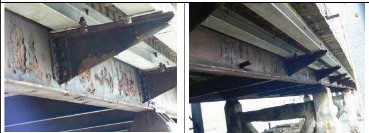
Chelsea Wharf – flaking of chlorinated rubber under-layer.
