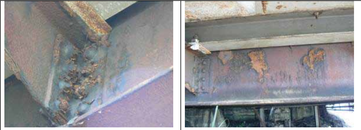
Chelsea Wharf – coating under Gold Seal exhibiting cracking and flaking on rivets and I-beams.
